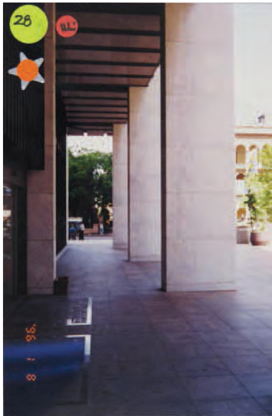
Figure 2.39 The view looking east along the colonnade facing Martin Place, with the Sydney Hospital in the background, prior to the construction of the podium addition.
